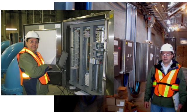
Mr. Amaury Pereira, P.Eng. RTS' Electrical Control Panel Specialist at the Control Room
