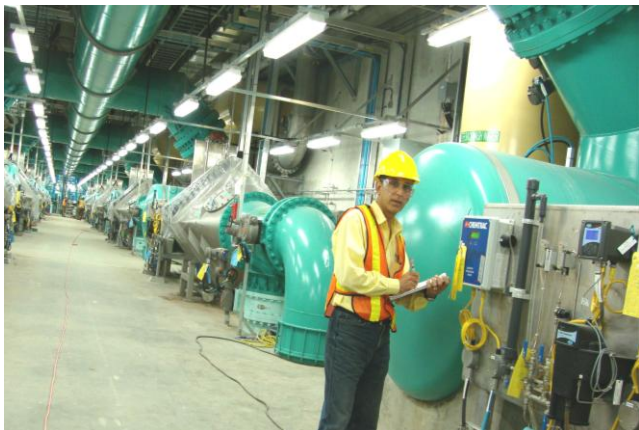
Mr. Mehran Abbasi, P.Eng. RTS' Instrumentation Specialist at the Filtration Area
