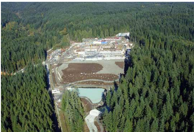
Aerial view of the filtration plant; it occupies a site of around 8 hectares, located in the Lower Seymour Conservation Reserve.
